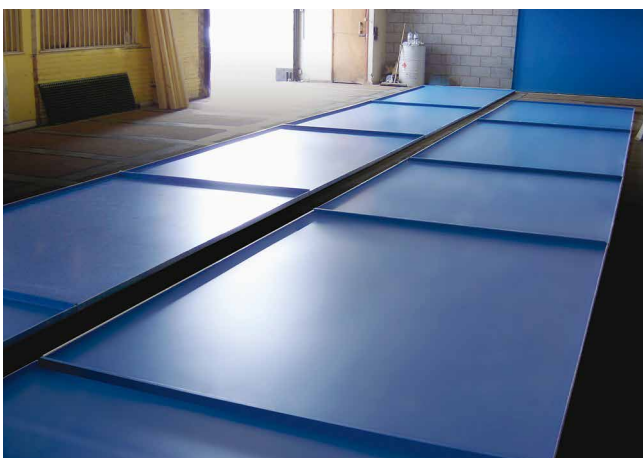
Large custom-built oil spill catchment bund for a manufacturing workplace.
